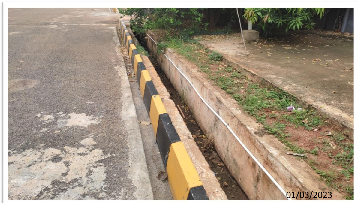
Storm water drainage Photograph
